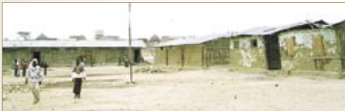
Ime School in poor condition
